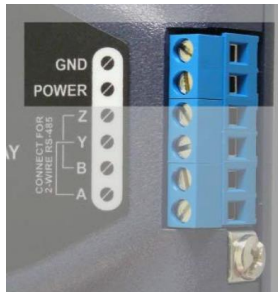
7VDC to 24VDC power terminals
